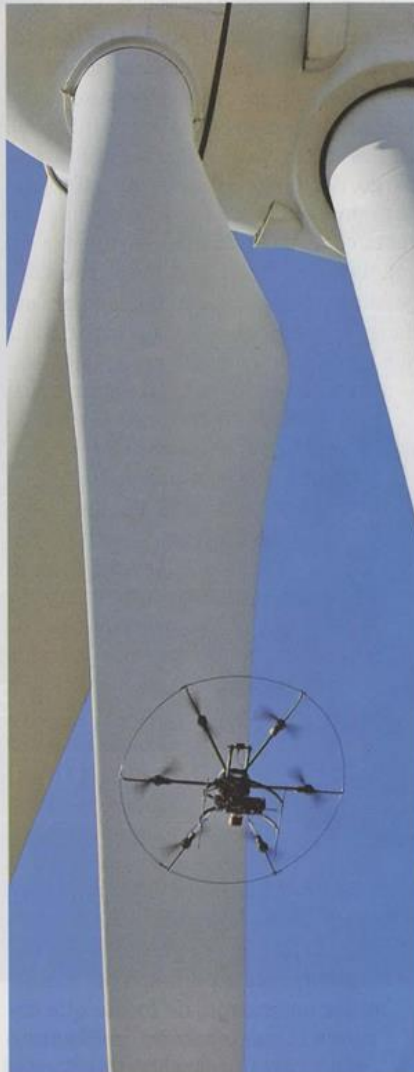
An Arborea Intellbird aerial device flies over an Iberdrola windmill to locate possible cracks
